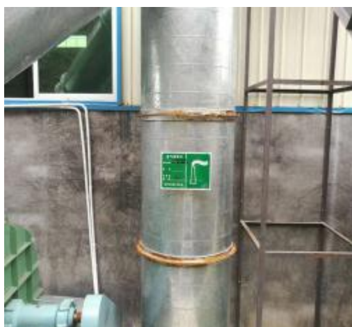
废气排放口标牌
